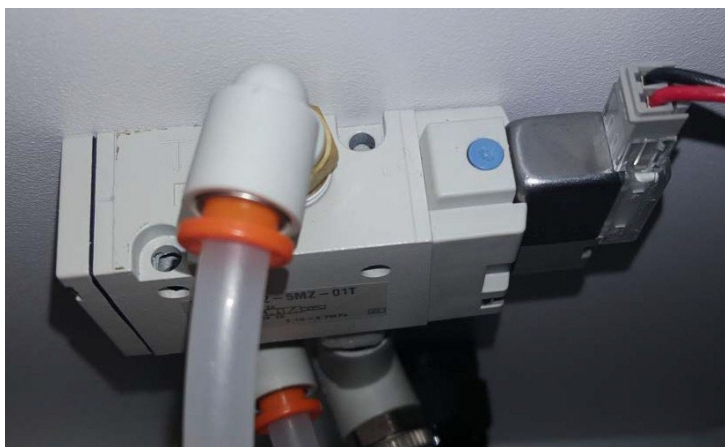
Figure 7-2: Isolation Valve Control Solenoid
