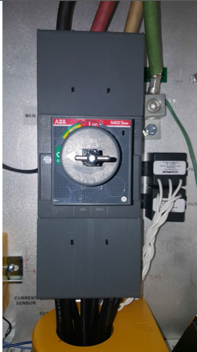
Figure 3-1: Main Circuit Breaker
